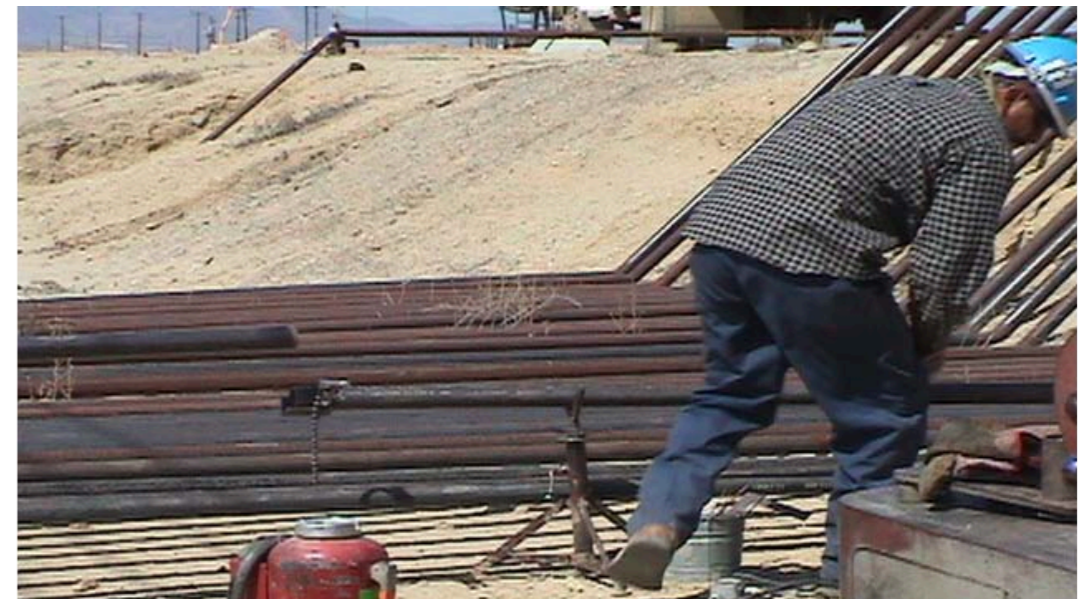
Limited space installation
