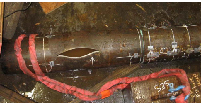
Figure 3: Pressure Containment Loss: Fish-Mouth Burst
